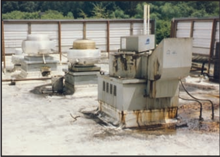
Grease Laden Rooftop
